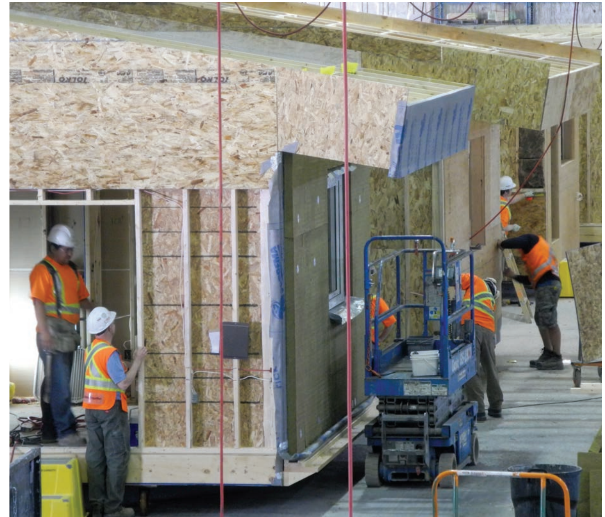
Bella Bella Passive House under construction in factory. Photo courtesy of Monte Paulsen, RDH Building Science
